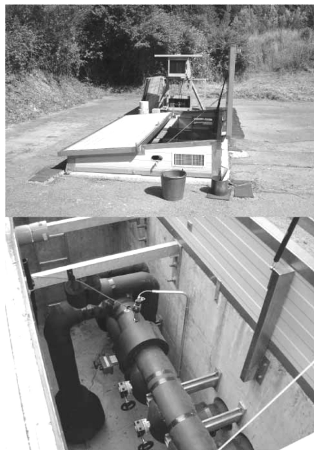
Figure 3.4: View of the P600 well head (photos taken during the water sampling for this study).
