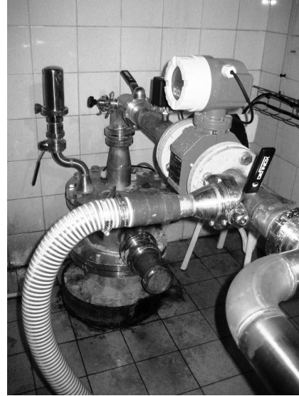
Figure 8.3: View of the Lépinay well head (February 2009).
