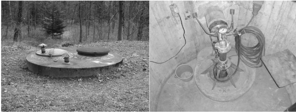
Figure 3.3: View of the P201 well head (photos taken by the Alpgeo consulting office).
